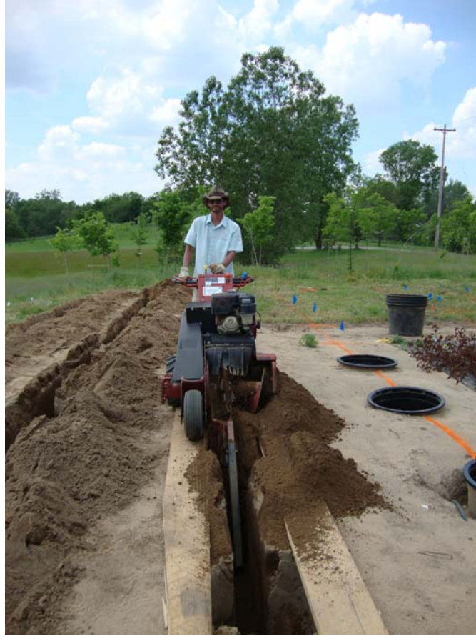
Photo 1. Research Technician Aaron Warsaw installs trenches for leachate collection system for MSU Pot-in-Pot research nursery
